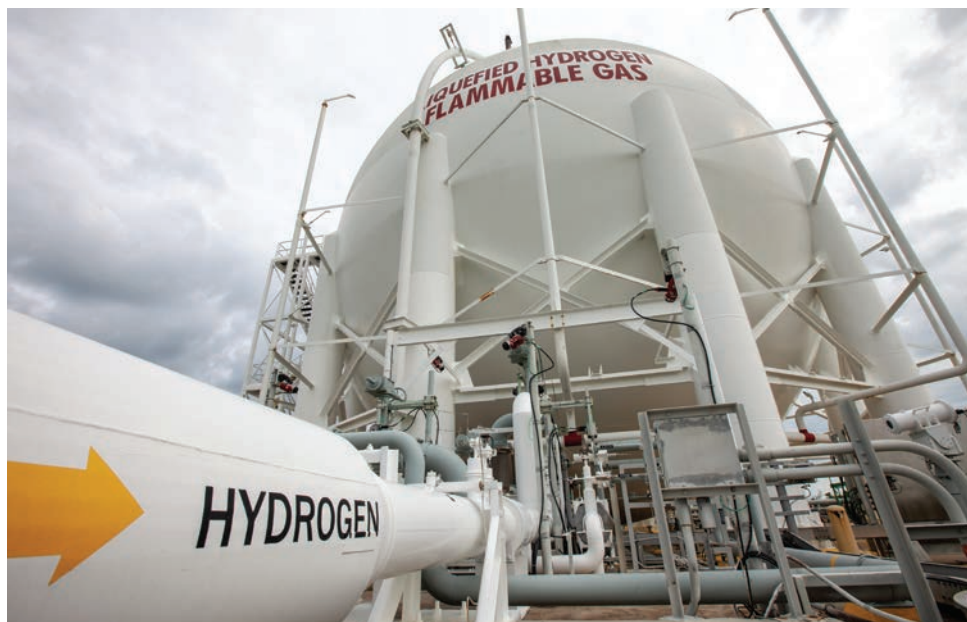
An 850,000-gallon liquid hydrogen storage sphere used to provide liquid hydrogen for rockets resides at NASA’s Kennedy Space Center.
