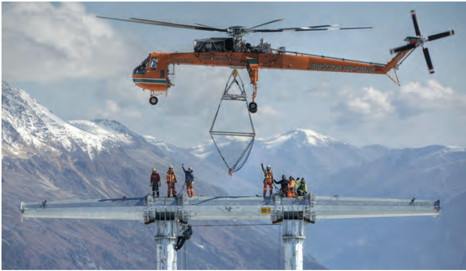
Powerline construction is just one of the many jobs facilitated by Erickson's S-64F helicopter.
